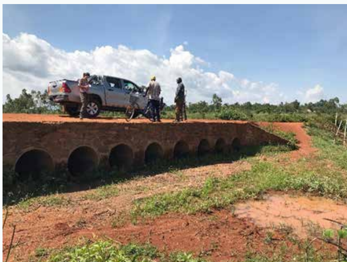
FIGURE 14. THIS TRIBUTARY OF THE RIVER SIO HAS NO RUNNING WATER AT THE END OF THE DRY SEASON OF EARLY 2019. HOWEVER, THE NUMBER AND SIZE OF THE CULVERTS UNDER THE ROAD SUGGEST MUCH HIGHER FLOWS DURING THE WET SEASON.
