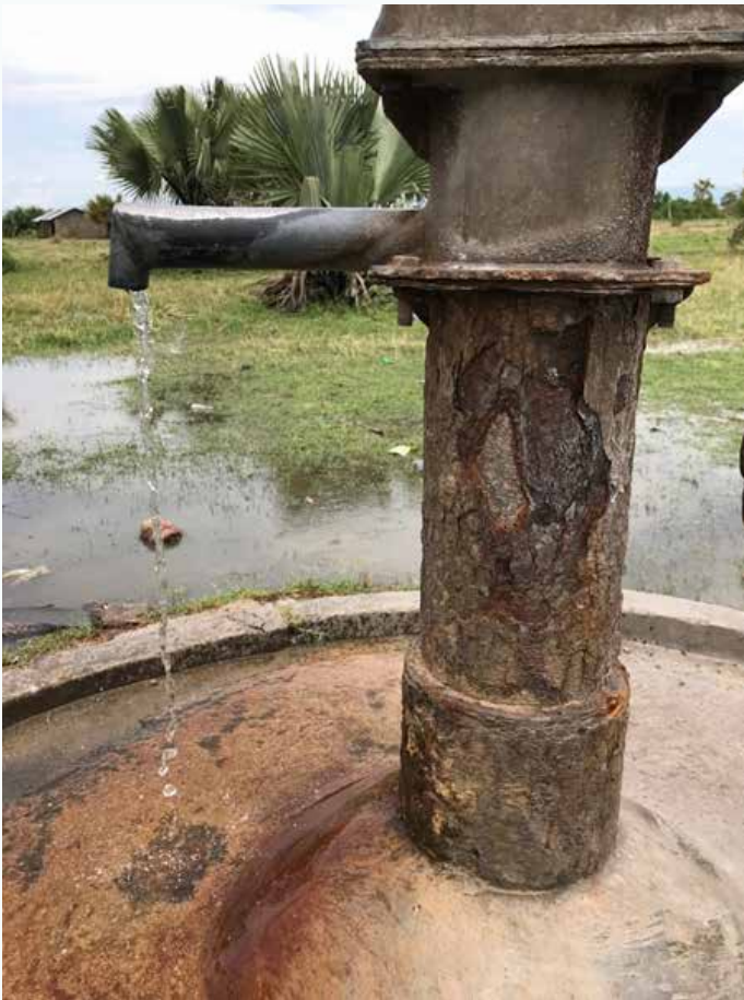
FIGURE 14: ABANDONED BUT STILL FUNCTIONAL PROTECTED WELL IN RWEBISENGO TOWN COUNCIL WITH CLEAR SIGNS OF CORROSION DUE TO THE HIGH SALT CONTENT OF THE WATER, LAT: 1°02'34.92"N / LON: 30°15'57.32"E.
