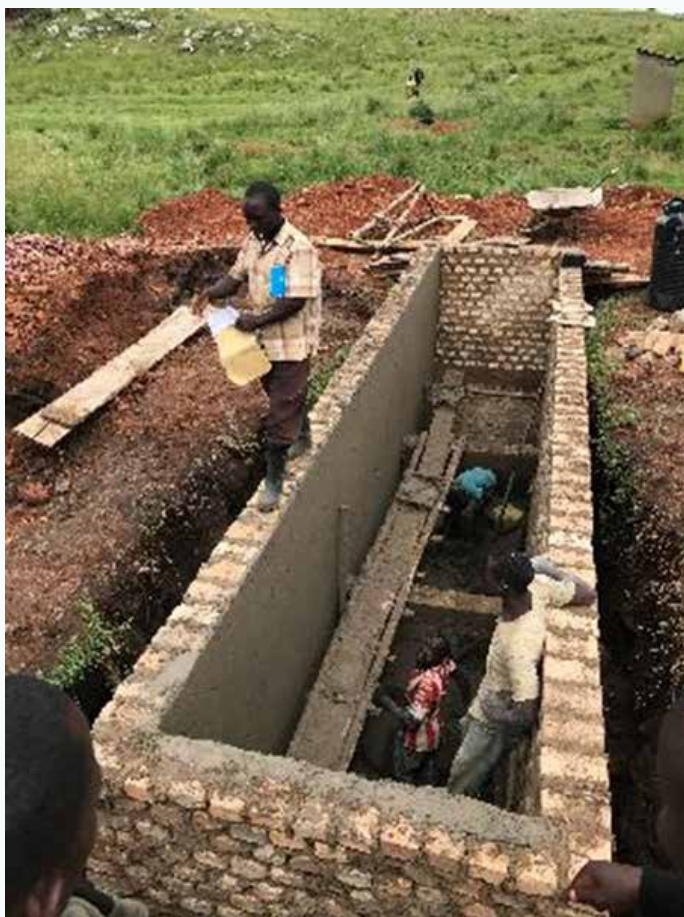
FIGURE 38: CONSTRUCTION OF A NEW 5 STAR VIP PUBLIC TOILET AT KASENSERO LANDING SITE. PHOTO TAKEN ON 27 APRIL 2019 AT LAT: 0°52'39.05" S / LON: 31°45'53.51" E.
