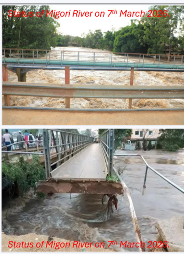
Figure 28: Traffic advisory on the closure by Highway Authority and the status of Migori Bridge on 7th March 2026.
