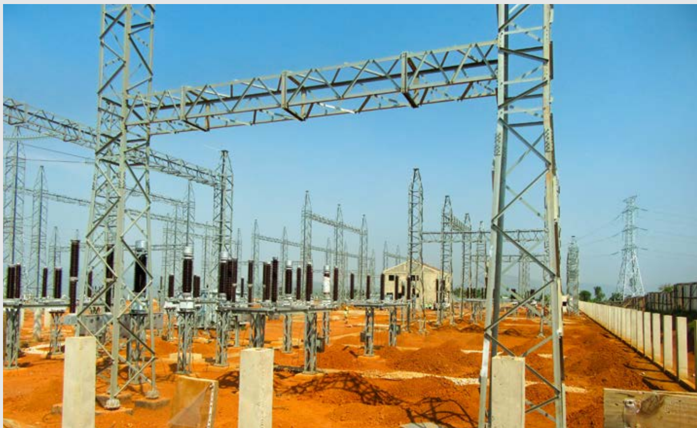
Shango power sub-station in Rwanda
