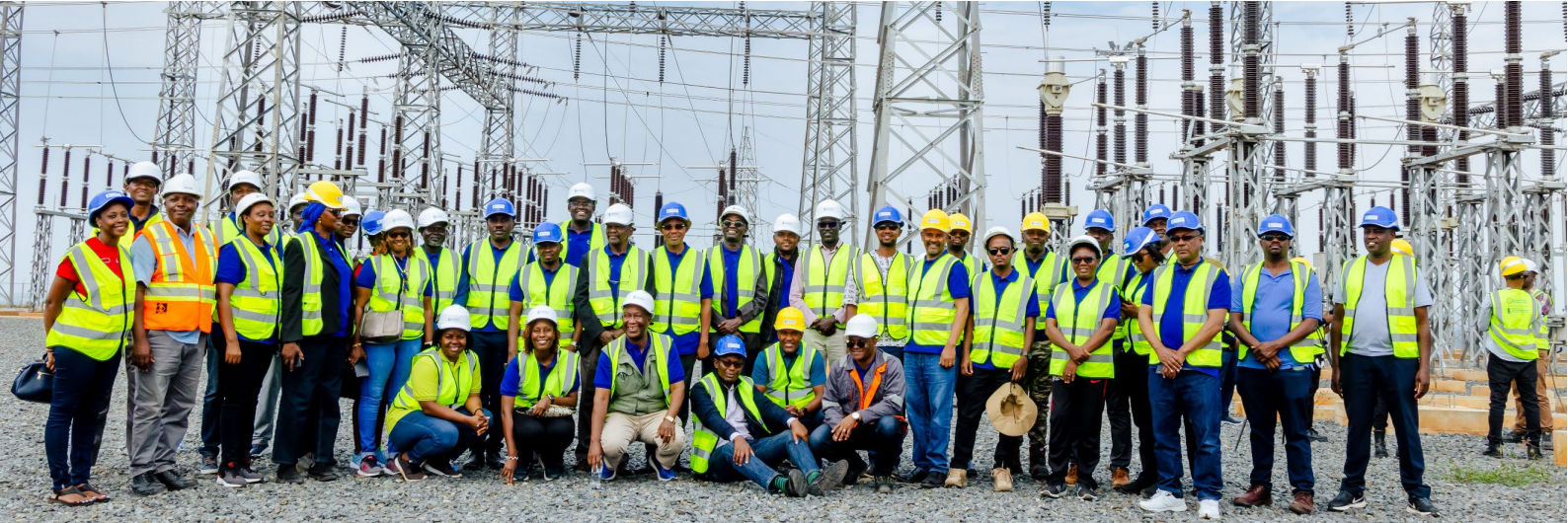
A delegation of Permanent Secretaries of the Ministries of Finance, Energy and Water of the NBI Member States visiting a Substation at the Rusumo Hydropower Project in Rwanda and Tanzania
