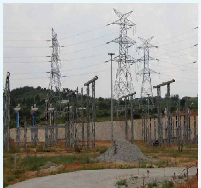
NELSAP WILL SUPERVISE CONSTRUCTION OF POWER SUBSTATIONS IN NGOZI AND GITEGA (BURUNDI) FOR EURO 6.79M AFDB FUNDING.
