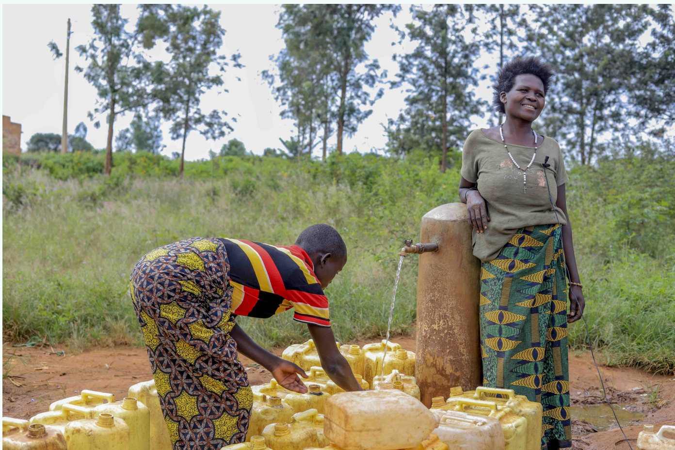
ONE OF THE COMMUNITY WATER POINTS AT THE BISHISHA WATER SUPPLY PROJECT
