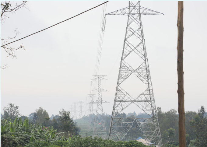
PART OF 160 KM RUSUMO-MUYINGA-GITEGA OVERHEAD TRANSMISSION LINE (OHTL) THAT ALSO INTERCONNECTS AND SYNCHRONIZES THE POWER GRIDS OF BURUNDI, RWANDA AND TANZANIA
