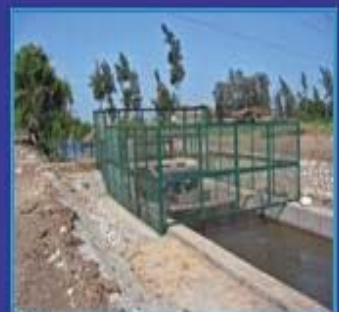
Automatic downstream water level control gate at intake
