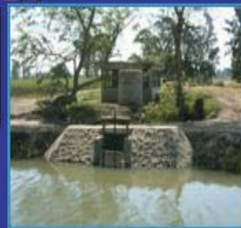
Single-point pumping station
