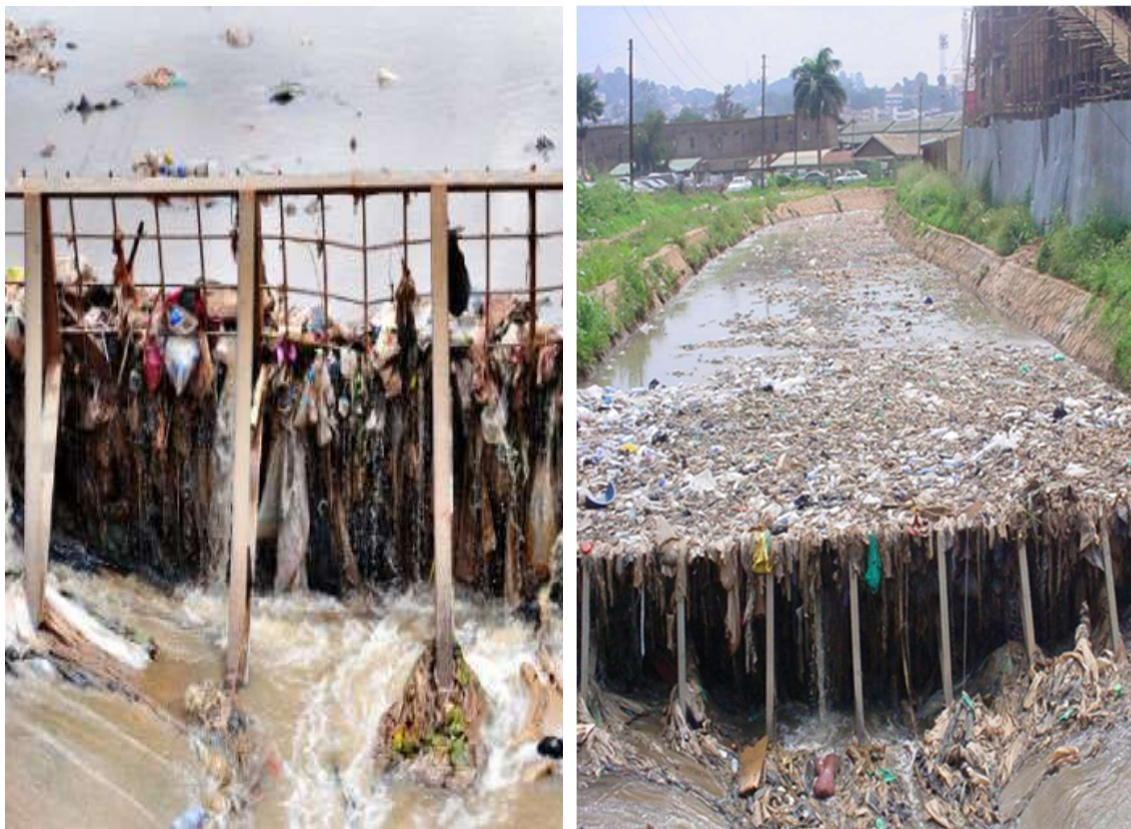
Figure 6.2: Kampala drainage channel choked by plastics. Source: Local expert (Uganda).
