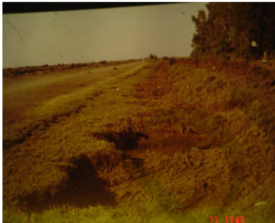
Plate (3) Inadequate Sedimentation Clearance of Irrigation Canal in GS
