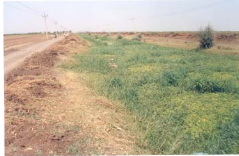
Plate (5) Aquatic Weeds Obstructing Water Flow in Irrigation Canal – Gezira Scheme
