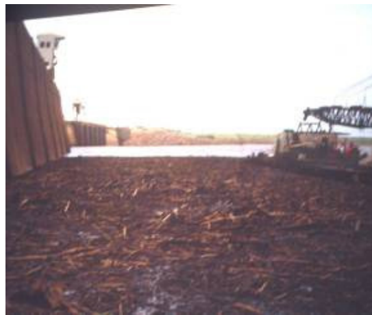
Plate (b) Debris in front of Turbines U/S Roseires Dam
