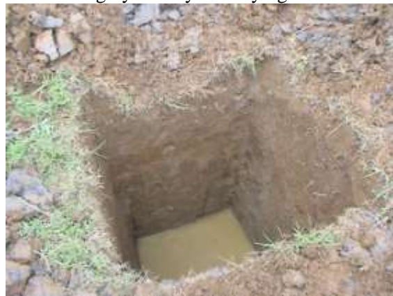
Figure 11: Black greyish clay overlaying the dam foundation
