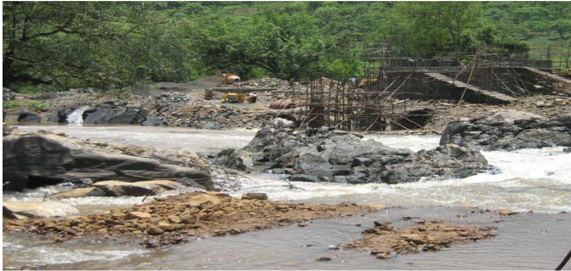
Figure 1.3 : The New Bridge Over Dedessa River is under construction (which means soon easy access to Chewaka and more population influx to the area)
