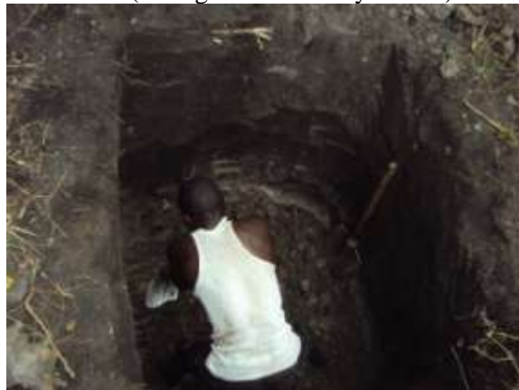
Figure 13: Geotechnical investigations on the 1st of April 2012 at Bigasha dam site (during the main rainy season)
