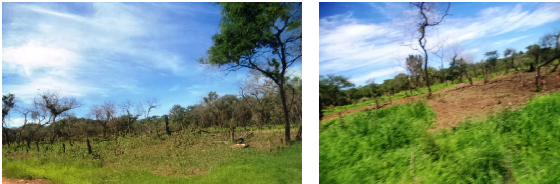
Figure 3-49: Clearing of wood land for the expansion of farm in Torit State, south Sudan
