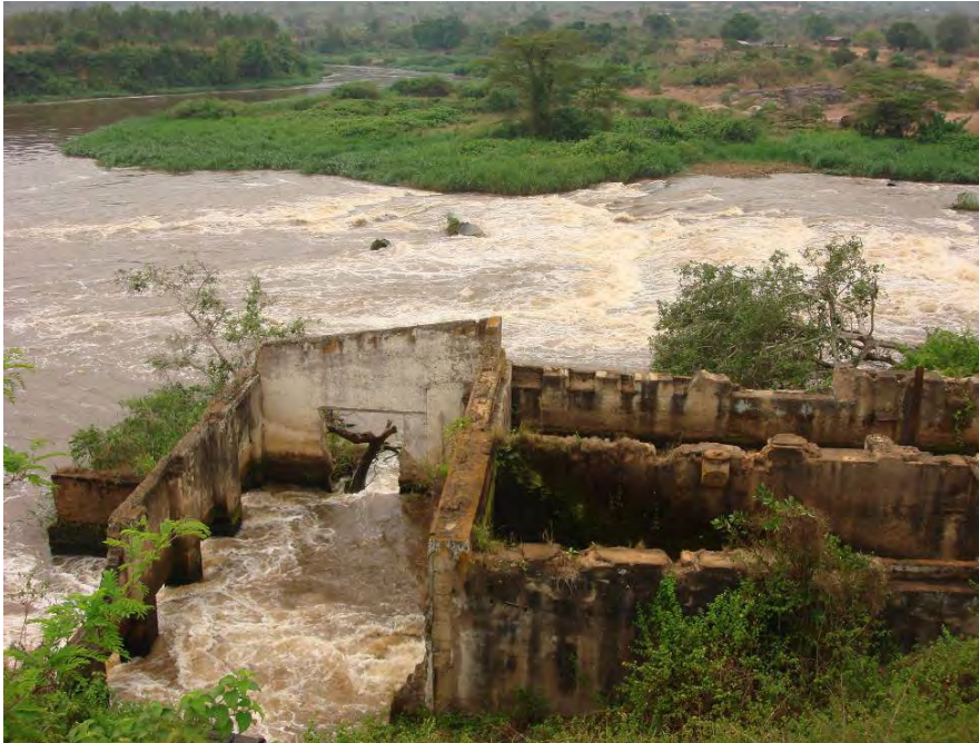
Figure 11: Ruins of the Power plant at Kikagati
